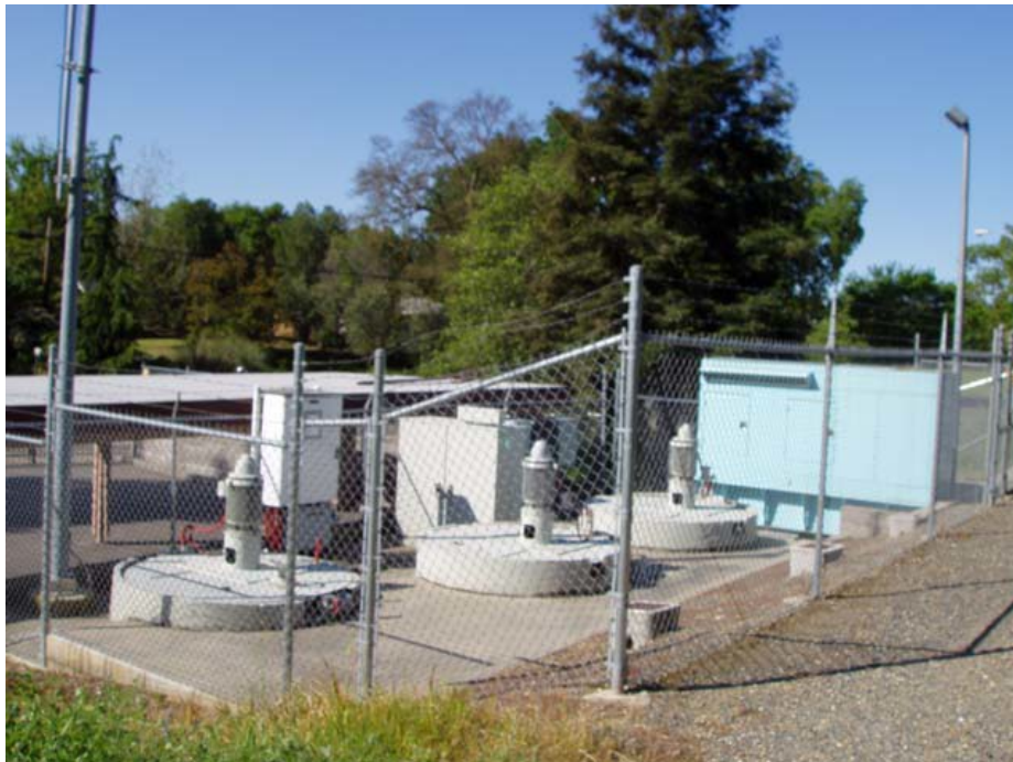
Figure 8 - D12 Winding Way Pump Station
